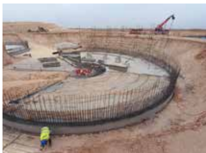
Station d'épuration Fqih Bensaleh
